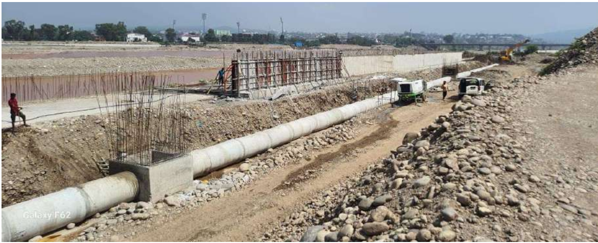
Picture showing Interceptor Drain On Left Bank
