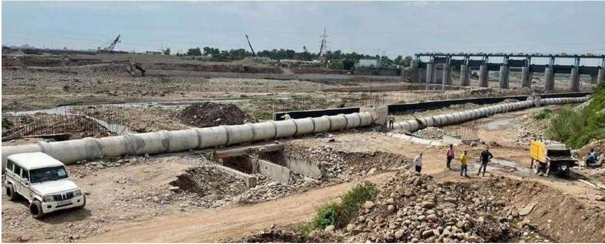
Picture showing Interceptor Drain On Right Bank
