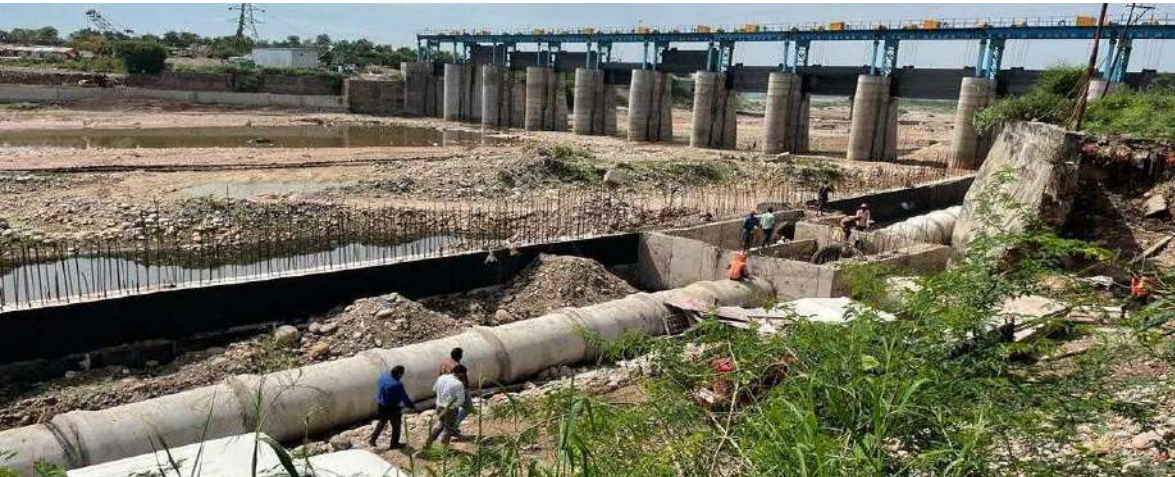
Picture showing Interceptor Drain On Right Bank
